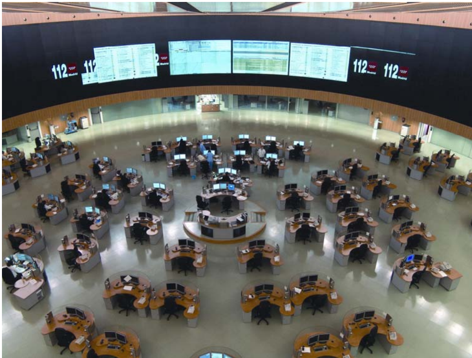
Figure 7. Alarm and command are coordinated at the 112 emergency call centre. 45 of the 90 switchboards are reserved for the police, rescue service, Samur and Summa 112 and Guardia Civil. Photo: Madrid 112
